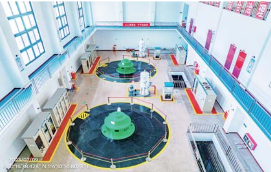
霍山县白莲崖水电站现代化厂房
